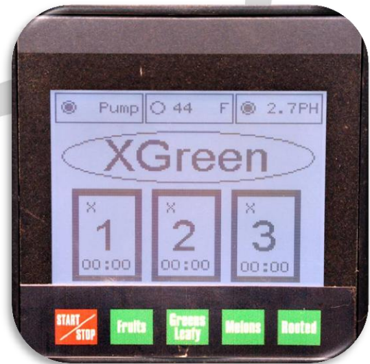
Figure 2: Operators can constantly monitor the temperature and pH on the X-Green control panel.
